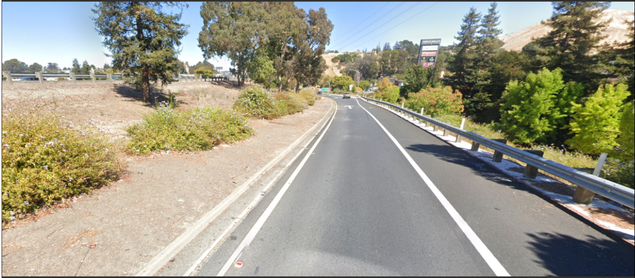
East-bound exit at creek over crossing (note the guard rail that allows trash to flow freely into creek)
