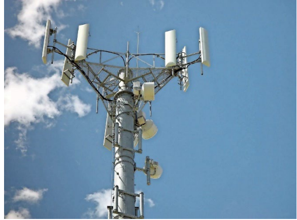
Figure 3 Typical 5G wireless antenna
