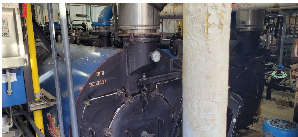
Figure C.21 Uninsulated boilers and pipes
