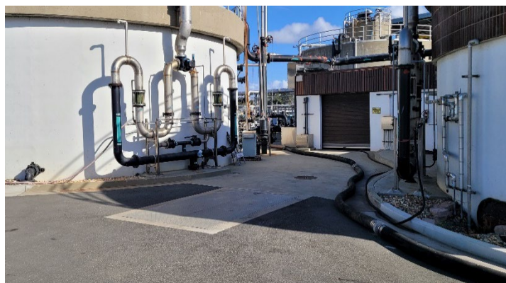
WWTP Anaerobic Digesters
