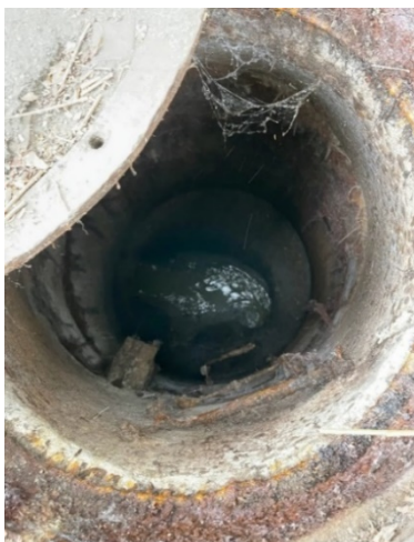
Figure 7 SSMH w/surface deterioration
