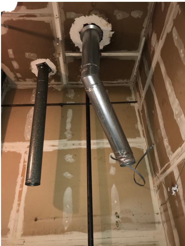
Photograph 32. Disconnected vents within former Four Mile Cleaners.
