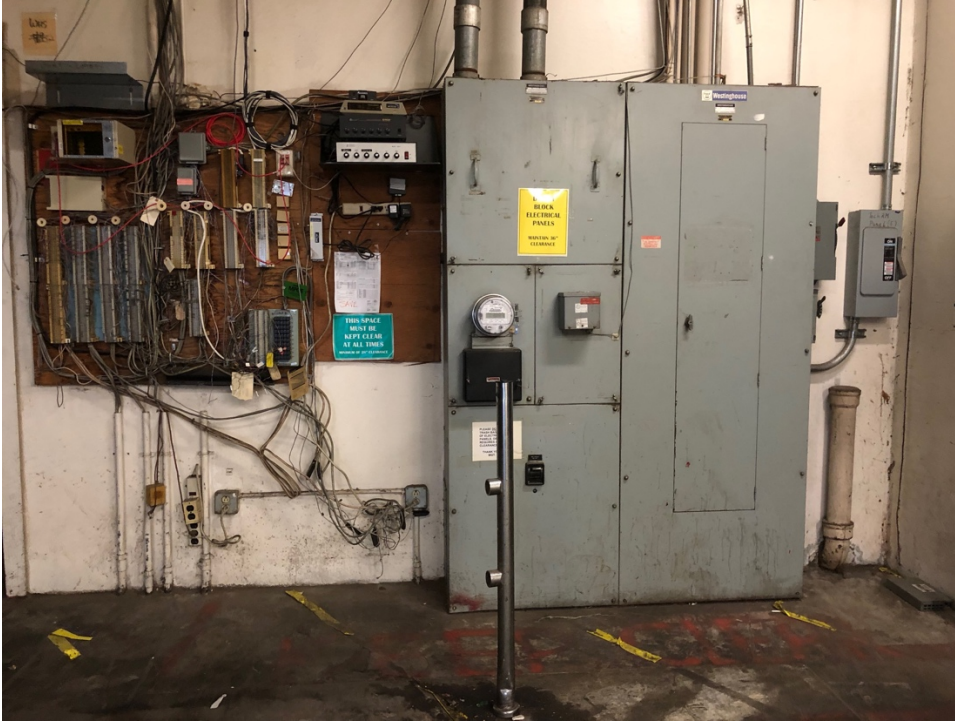
Photograph 23. Electrical control panel within former CVS Pharmacy.
