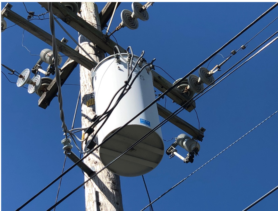
Photograph 17. Pole-mounted transformer labeled “non-PCB”.
