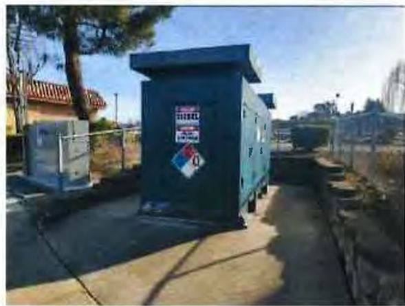
14. View of the West County Wastewater emergency generator, equipped with a 200-gallon AST, observed adjacent to north-northeast.
