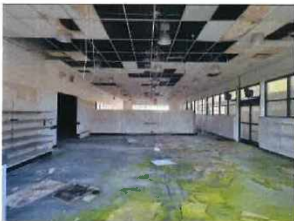
5. View of the internal condition and water damage observed through a glass door on the northeast portion of the building in the subject property.
