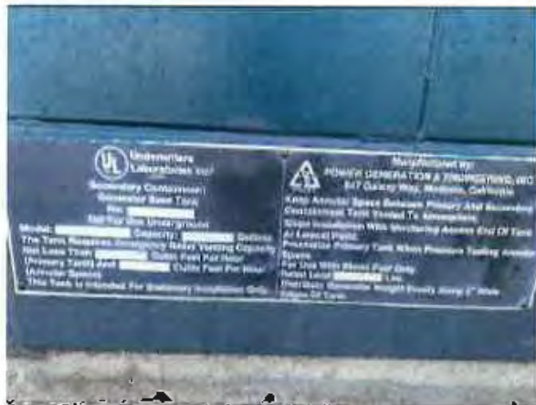
15. View of the plate identifying the emergency generator and associated belly tank observed adjacent to the north northeast.
