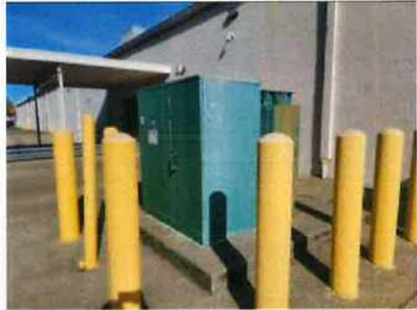
10. View of one electrical transformer observed on the west side of the subject property.
